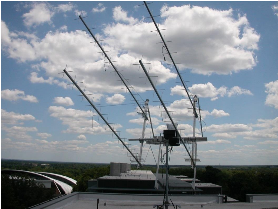
Fig. 1. – Four-Yagi dual-polarization 432 MHz array at W2PU. The Yagis are rear-mounted; boom length is 3.5 m, and stacking distance is 1.2 m in each direction.
